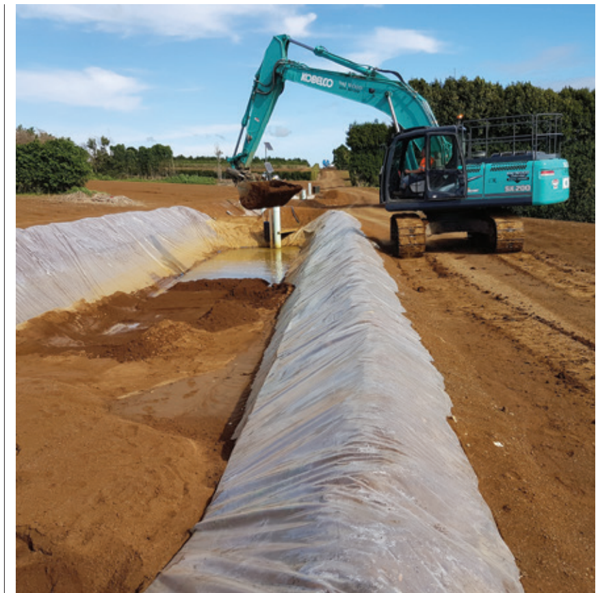
Sediment traps being cleaned following an extremely wet March 2017 – Don't Muddy the Water project.
