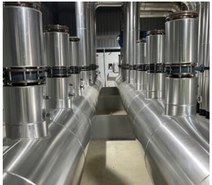
A hot water buffer tank system with precise controllers and insulated pipework to optimise heat efficiency by more than 25%
