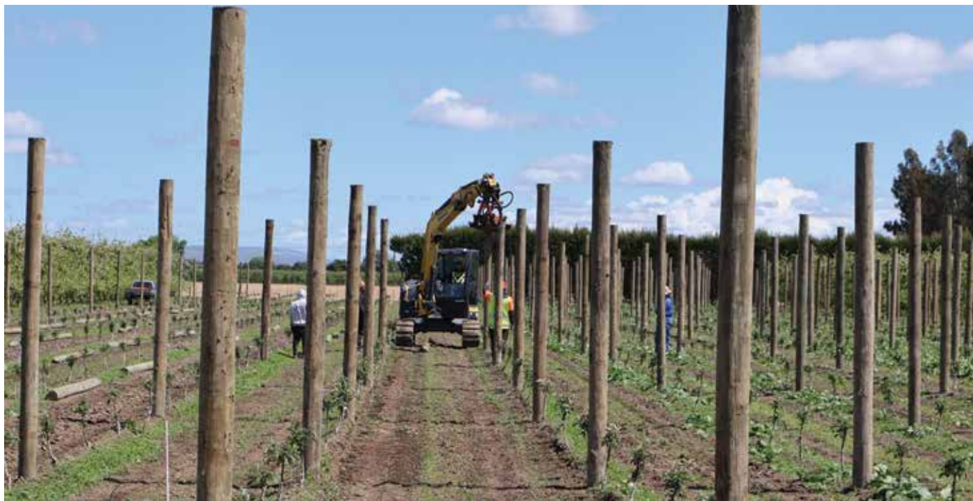
It's a tight fit for the machinery, but all new plantings at the Shearers orchard are spaced at 2.5 metres, including their new Joli trees
